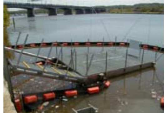
FLOATING CSO TRASH NETTING SYSTEM ON THE TIDAL RIVER (DISTRICT OF COLUMBIA)
