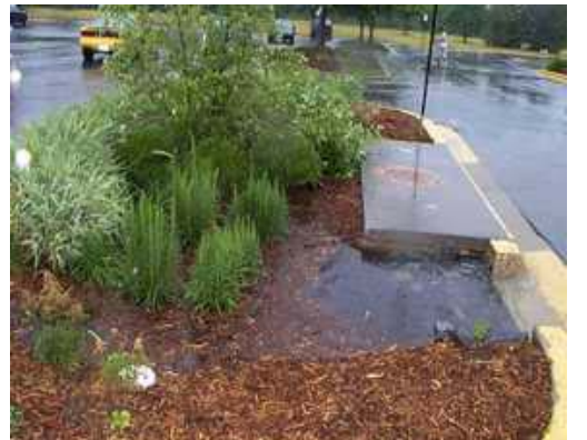
RECENT BIORETENTION STORMWATER SYSTEM INSTALLED IN PRINCE GEORGE'S COUNTY
