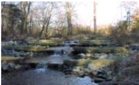
COMPLETED PAINT BRANCH STEP POOL FISH PASSAGE PROJECT AT MAYDALE NATURE CENTER
