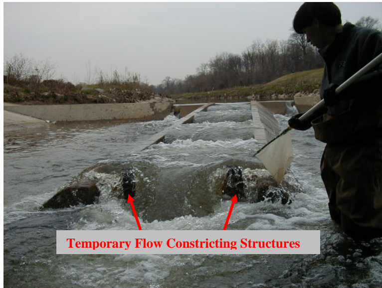
Figure 9. Temporary Repair at the Lowest Downstream Baffle on the Northwest Branch fishway at US Route 1
