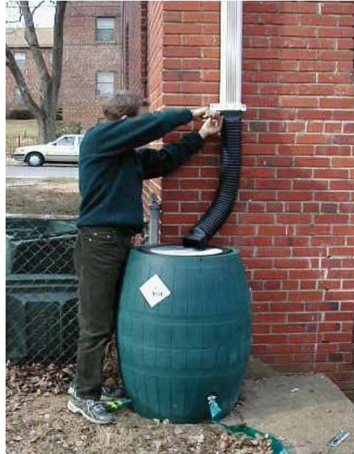
Figure 8. Rain Barrel Installation at Site No. 10
