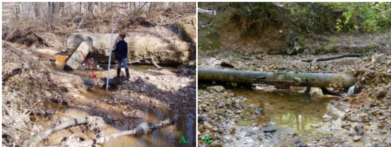
Figure 11 - A. Middle Reach - Exposed Three Foot Long 10" DIP Section , May 2004; B. Middle Reach - Exposed Eight Foot Long 10" DIP , October 2004
