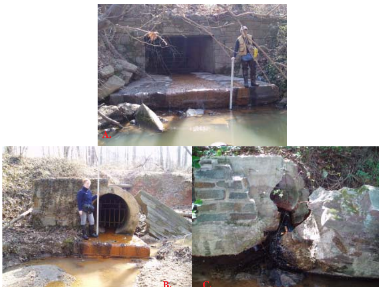
Figure 2 - Fort Chaplin Tributary - A. Texas Avenue Storm Drain Outfall (4' high by 8' wide concrete box culvert); B. East 'D' Street Storm Drain Outfall (48" RCP); C. West 'D' Street Storm Drain Outfall (27" RCP)
