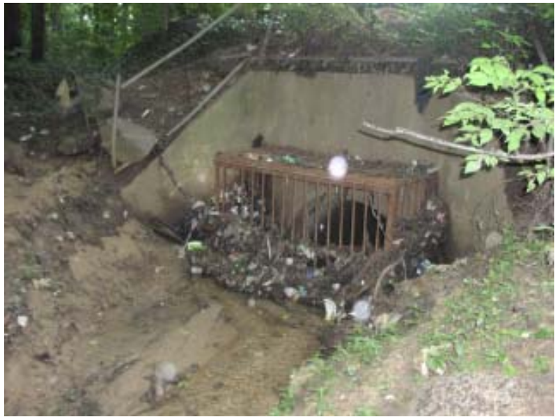
Figure 34 - Lower Reach - 'C' Street 48" RCP - Debris/Trash Filled Rack
