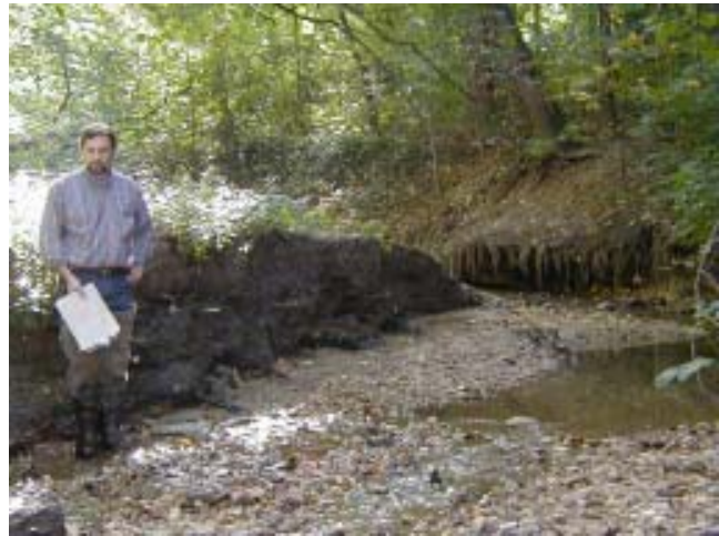
Figure 28 - Lower Reach - Severe Channel Erosion
