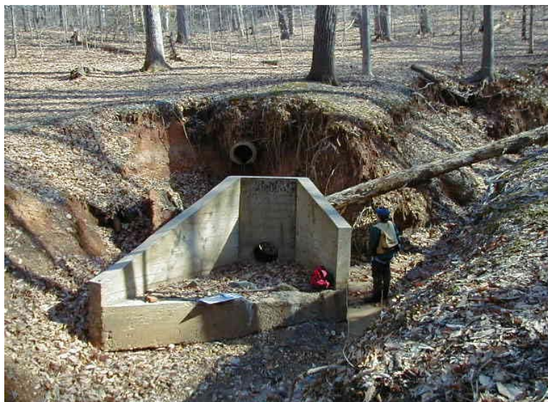
Figure 9. Upper Mainstem: Broken Concrete Storm Drain Outfall Apron (X-2 area)
