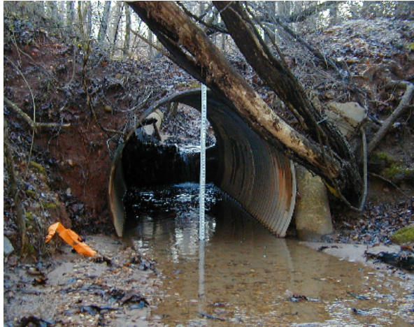
Figure 16. 78" CMP with 3' Drop at Upstream End (X-12)
