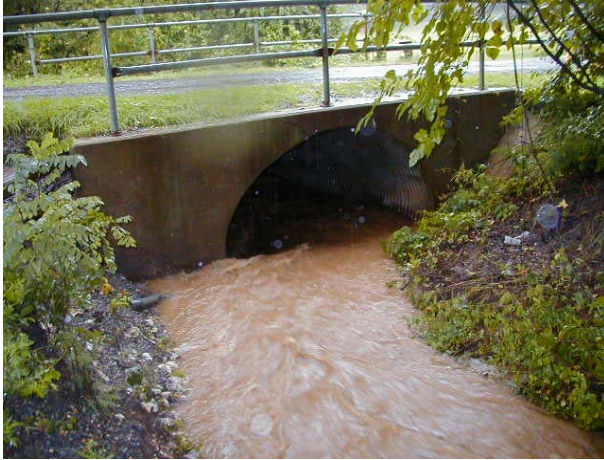
Figure 29. Hurricane Floyd: NPS Maintenance Road Culvert Looking Downstream (X-19 area)
