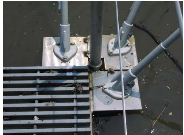
Figure 29. Vulnerable 'Outrigger' Mounting Brackets
