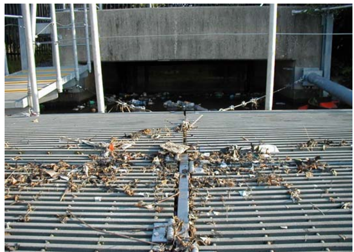
Figure 26. Debris on Upper Surface of Netting System Deck as Evidence of Submergence During Periods of Heavy CSO Flow and/or Tidal Action
