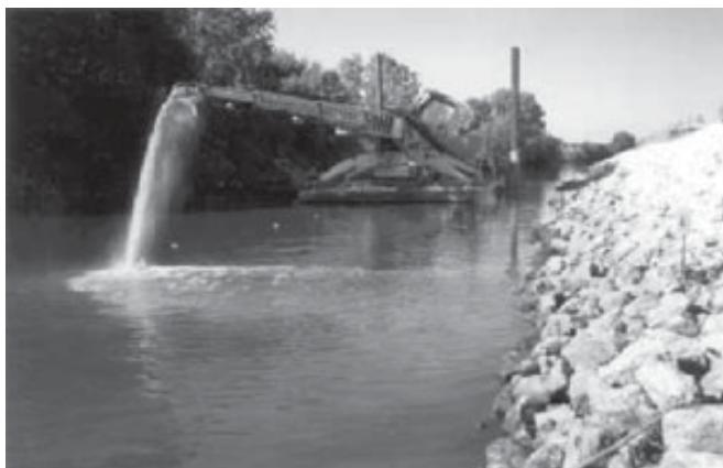
MEASURES SUCH AS THE CONSTRUCTION OF A REACTIVE CAP SHOULD GREATLY REDUCE THE MOVEMENT OF TOXINS FROM RIVERBED SEDIMENTS INTO THE WATER COLUMN
