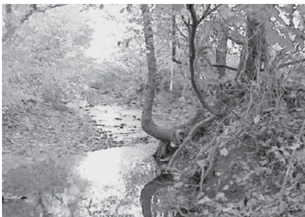
STREAM BANK EROSION ALONG CAMPUS CREEK, ONE OF SEVERAL SITES SCHEDULED FOR RESTORATION ON THE COLLEGE PARK CAMPUS
