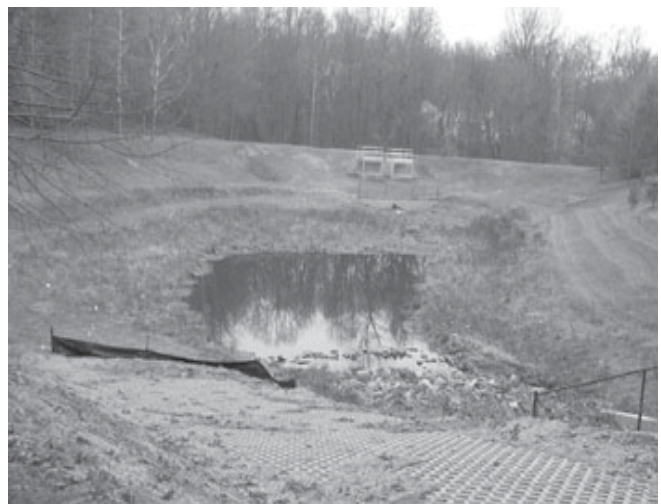
SNOWDENS MILL STORMWATER MANAGEMENT FACILITY
