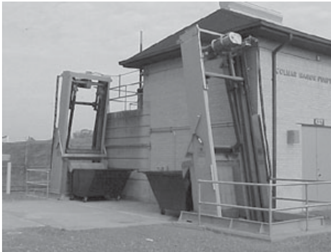
THE RECENTLY INSTALLED AUTOMATED TRASH REMOVAL SYSTEM AT THE COLMAR MANOR PUMP STATION
