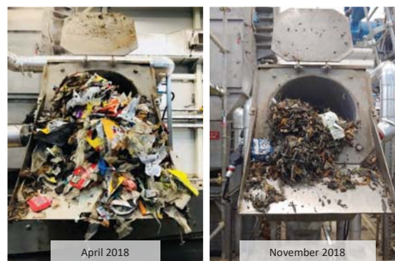
Trash and debris removed from CSO captured by tunnel at ECF Fine Screens
